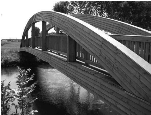
Figure 7. Metal caps and larch cladding are used to protect the main untreated spruce glulam members of this bridge near Aachen, Germany.
