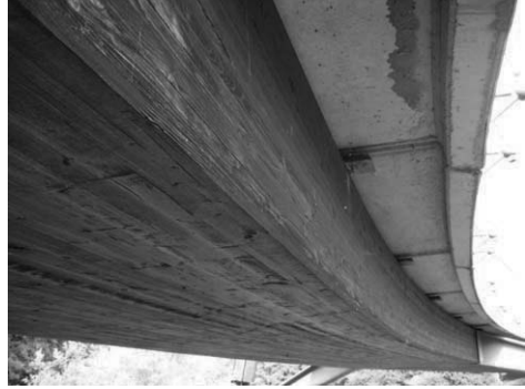
Figure 6. In this bridge at Wernau, Germany, the untreated spruce glulam is protected from wetting by the overhanging precast deck.
