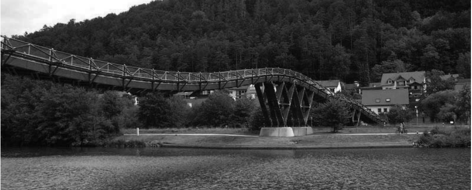
Figure 4. The famous ribbon bridge at Essing relies on in-situ finger joints to form the continuous glulam beams, which are protected by the wooden deck.
