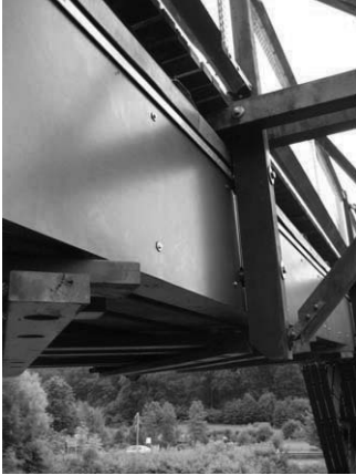
Figure 5. Detail of Essing showing the protective cladding that has recently been added to the sides of the ribbon beams.
