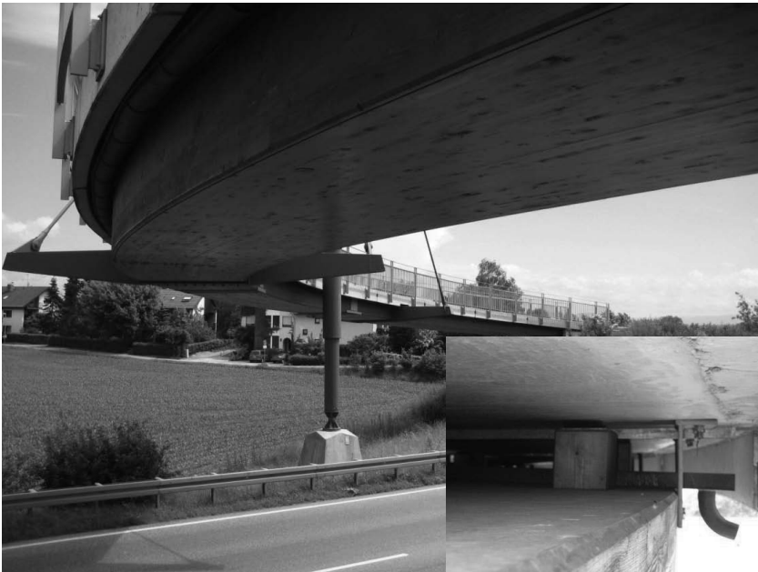
Figure 8. This bridge at Hochstetten, Germany improves on the details at Wernau – as shown in the detail the top of the timber is laid to falls and a sufficiently large ventilation cavity is provided above to allow future inspection.
