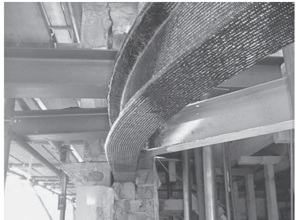
Fig. 43.8 The upgrading of a curved steel structural beam by the carbon fibre/epoxy composite low-temperature mould prepreg (Courtesy of Taylor Woodrow, UK, and ACG Derbyshire, UK).
