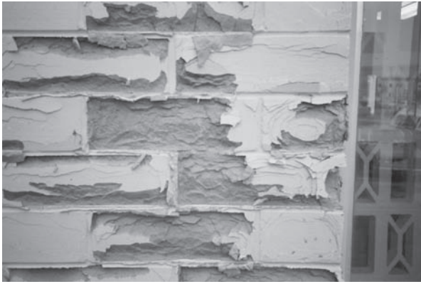
Fig. 37.4 Erosion due to frost attack.
