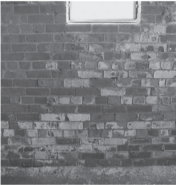
Fig. 37.5 Salt crystallisation damage to masonry together with associated soluble salt crystals (efflorescence).
