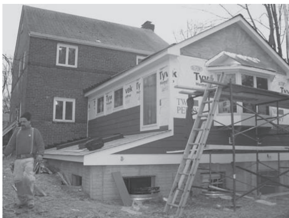
Fig. 50.5 Natural-FRC sidings being installed. (Photo by Mark Zimmerman, US (2007), reproduced from flickr.com/photos/pdz_house under Attribution 2.0 Generic License (see creativecommons.org for license details).)
