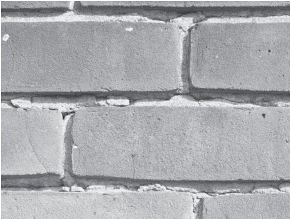
Fig. 37.2 Sulphate attack on mortar.
