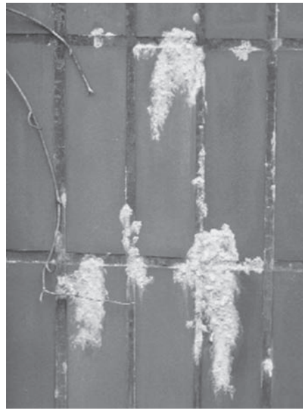
Fig. 37.6 Lime staining of brickwork.
