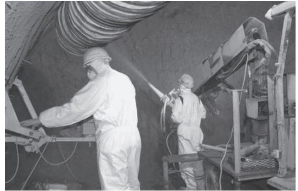
Fig. 50.3 Tunnel lining (steel-FRC) spraying equipment. Note the segmental extendable arm (top right, in partially retracted position) and computer control systems for laser guidance and monitoring (left). (Reproduced from the presentation accompanying Eddie and Neumann, 2004, by kind permission of the authors and Morgan Est Ltd/Beton-und Monierbau.)
