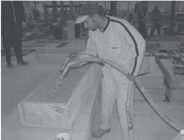
Fig. 49.2 Spraying of premix glass-FRC. (Supplied by Iain D. Peter, Powersprays Ltd., UK ( www.power-sprays.co.uk )).
