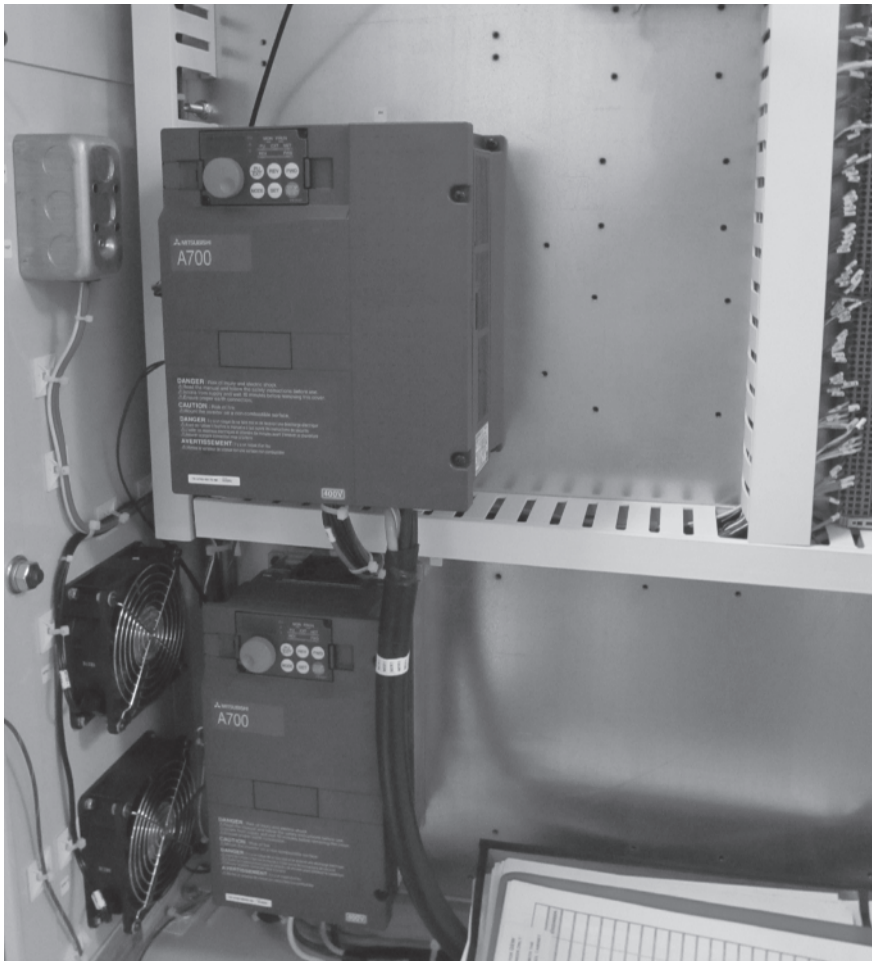
FIGURE 15-1 Solid-state motor controllers mounted in cabinets.
