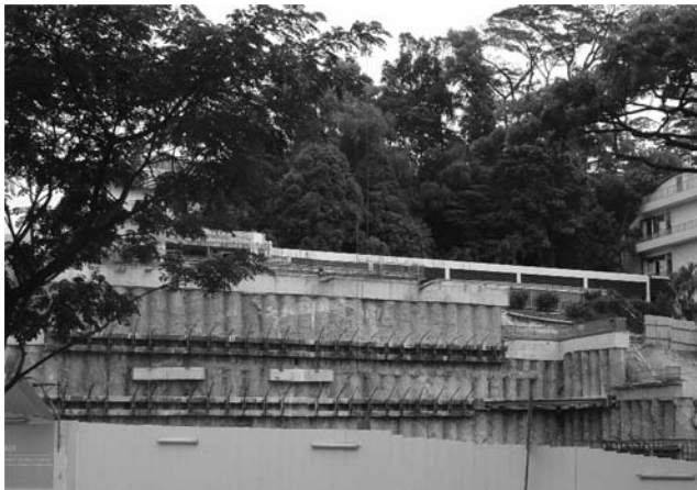
Figure 6.10 Braced excavation at National University of Singapore campus using contiguous-bored concrete piles with tieback support. (Courtesy of An-Bin Huang, Hsinchu, Taiwan.)
