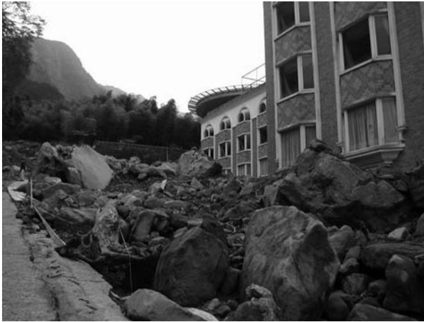
Figure 9.5 Debris flow during Typhoon Toraji in 2001 nearly destroyed a hotel in Nan-Tou, Taiwan. (Courtesy of An-Bin Huang, Hsinchiu, Taiwan.)
