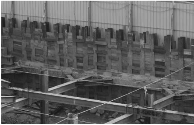
Figure 6.3 Soldier pile wall and its lateral support system. (Courtesy of An-Bin Huang, Hsinchu, Taiwan.)
