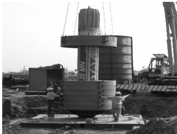
Figure 8.45 Field setup of the Statnamic load test. (Courtesy of DECL, Taipei, Taiwan.)
