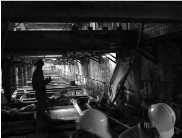
Figure 6.7 Cross-lot bracing of a cut-and-cover excavation for a subway station of Kaohsiung MRT project, Taiwan. (Courtesy of An-Bin Huang, Hsinchu, Taiwan.)
