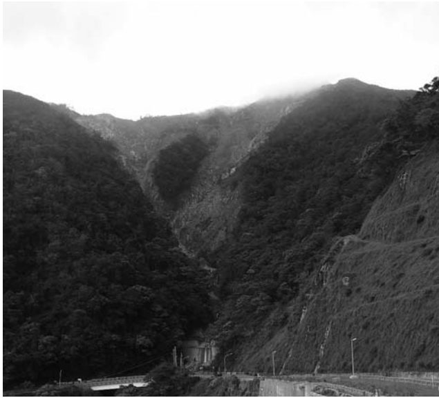
Figure 9.2 Scar created by a fatal landslide along Su-Hua Highway after typhoon Megi. (Courtesy of An-Bin Huang, Hsinchu, Taiwan.)
