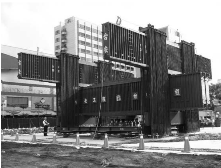
Figure 8.35 Pile load test using a reaction frame with 75,000 kN capacity. (Courtesy of DECL, Taipei, Taiwan.)
