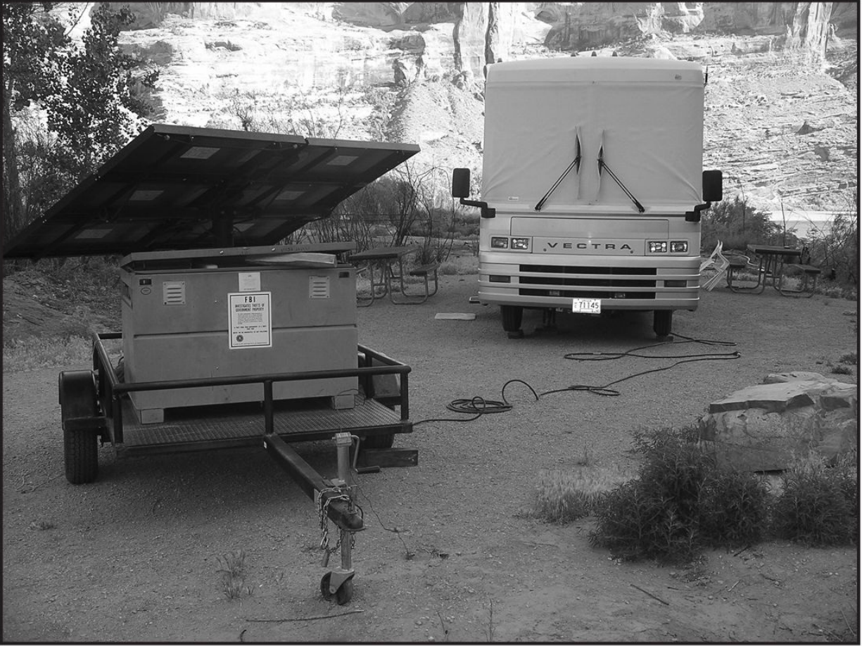
Solar array mounted on a trailer. Note the ground wire leading from the system and spiked into the earth near the trailer hitch.
