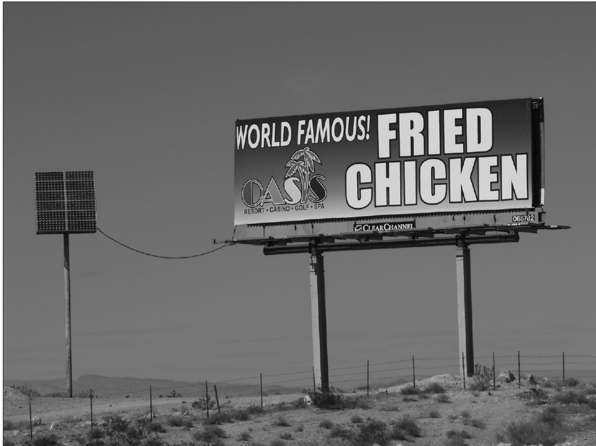
Pole-mounted panels powering billboard lights.
