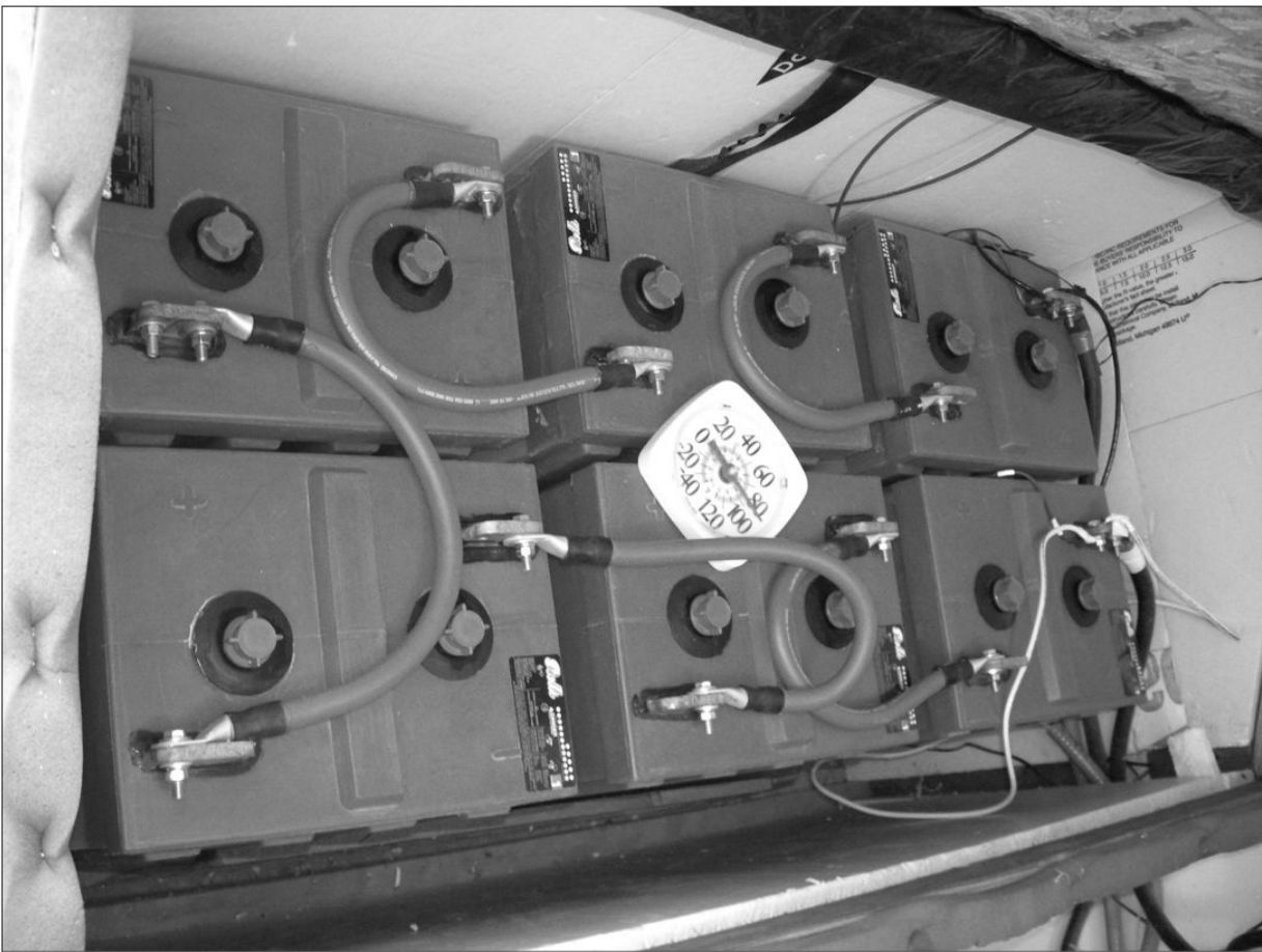
Six, 4-volt 1325 AH batteries wired in series to produce 24 volts.
