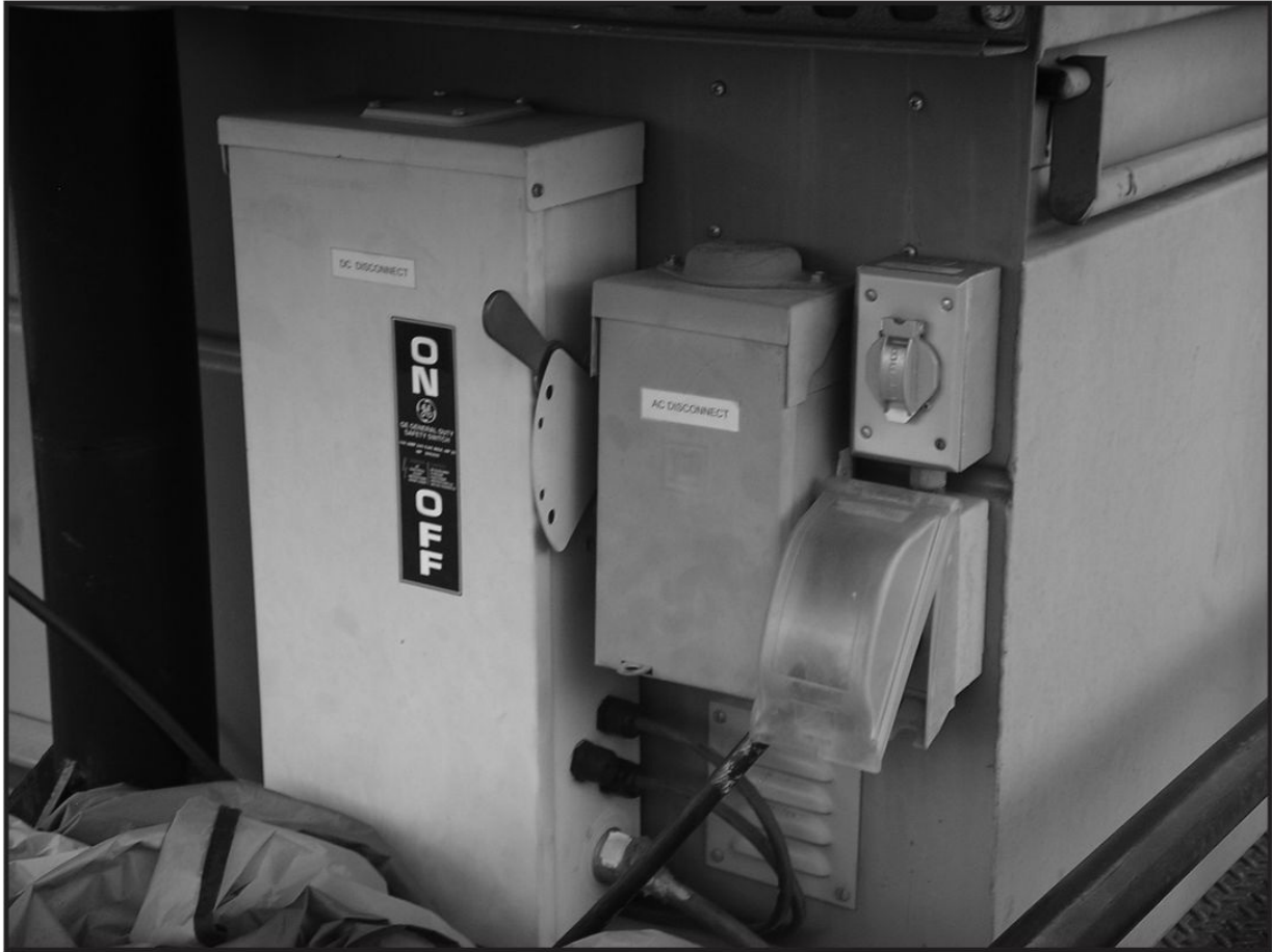
AC and DC disconnects and receptacles, mounted on the rear of the box.
