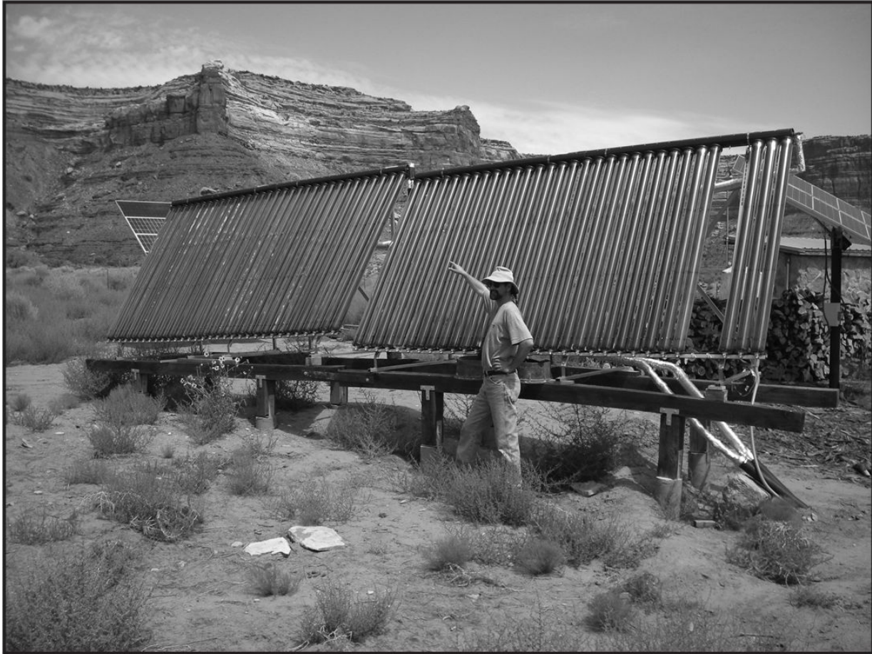
Evacuated tubes: This evacuated tube system at Valley of the Gods B&B provides hot water for the owners and four guest rooms.
