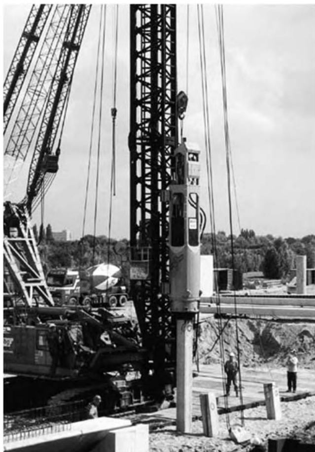
Figure 3.14 BSP CX110 hydraulic piling hammer on Hitachi crane-mounted leader (courtesy BSP International Foundations Ltd).
