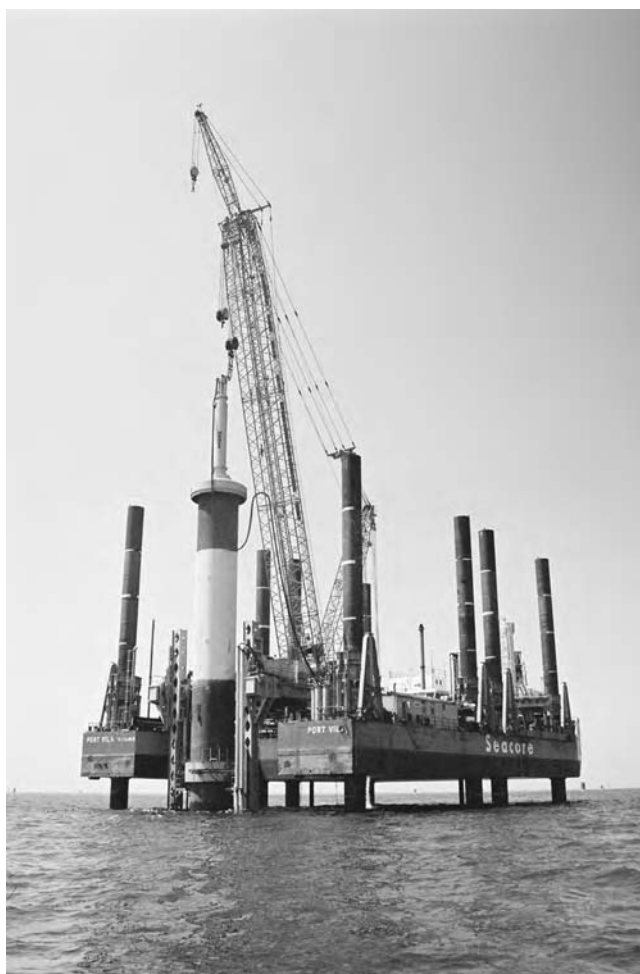
Figure 3.13 Driving a 4 m dia monopile foundation for North Hoyle offshore wind farm using a Menck MHU 500T hammer with large diameter pile sleeve and anvil adapter (courtesy Seacore Ltd).
