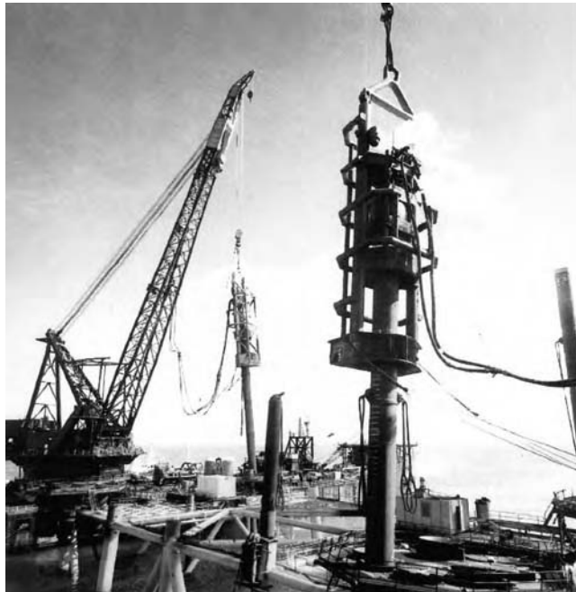
Figure 3.12 MRBS air/steam single-acting hammer with stabilizing cage driving 54 inch diameter piles in legs of offshore jacket platform (courtesy Menck GmbH).
