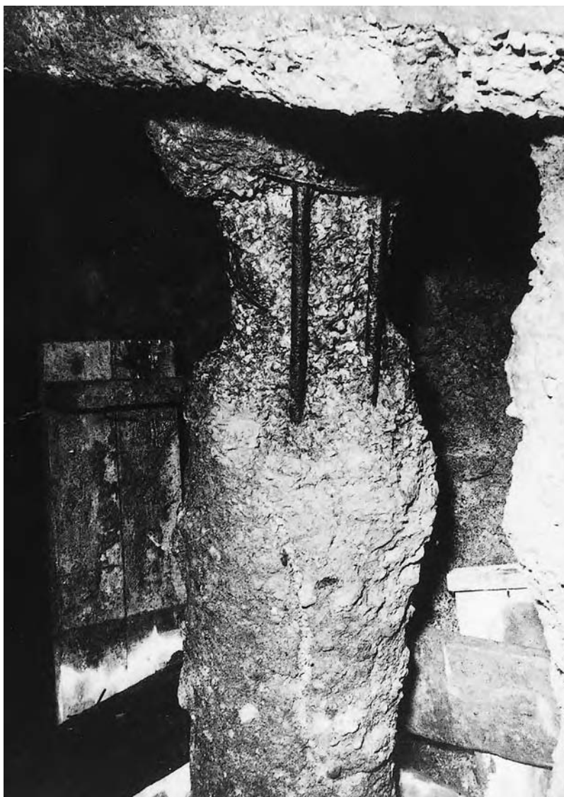
Figure 10.3 Disintegration of concrete in bored and cast-in-place pile due to attack by sulphuric acid leaking into fill from industrial processes.
