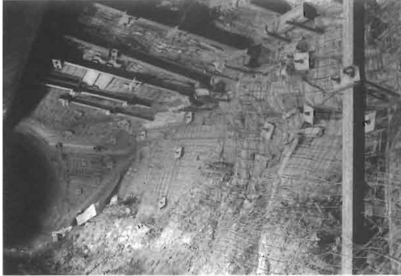
Figure 2.6 Tunnel in mudstone which has deteriorated over a period of several years after excavation.
