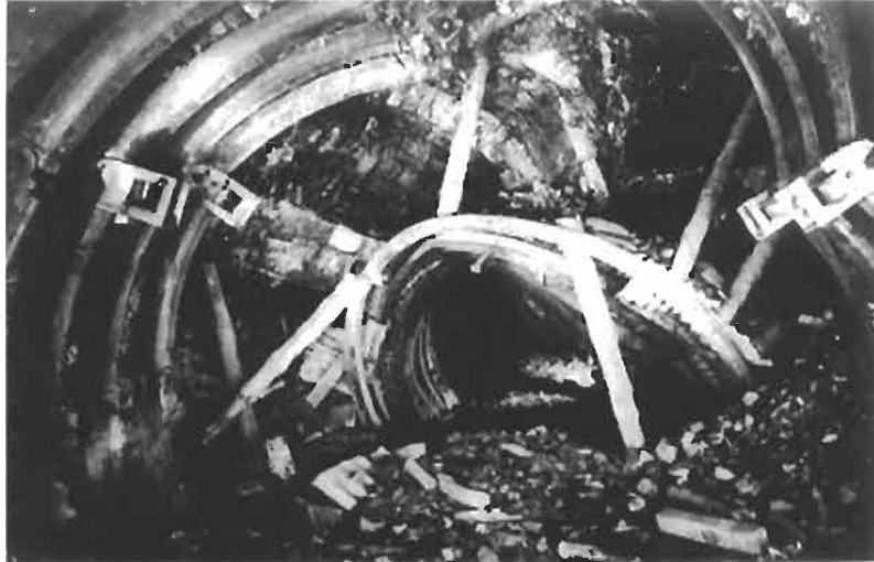
Figure 5.1 Large displacements around an originally arch-shaped coal mine access tunnel (from Pan, 1989).
