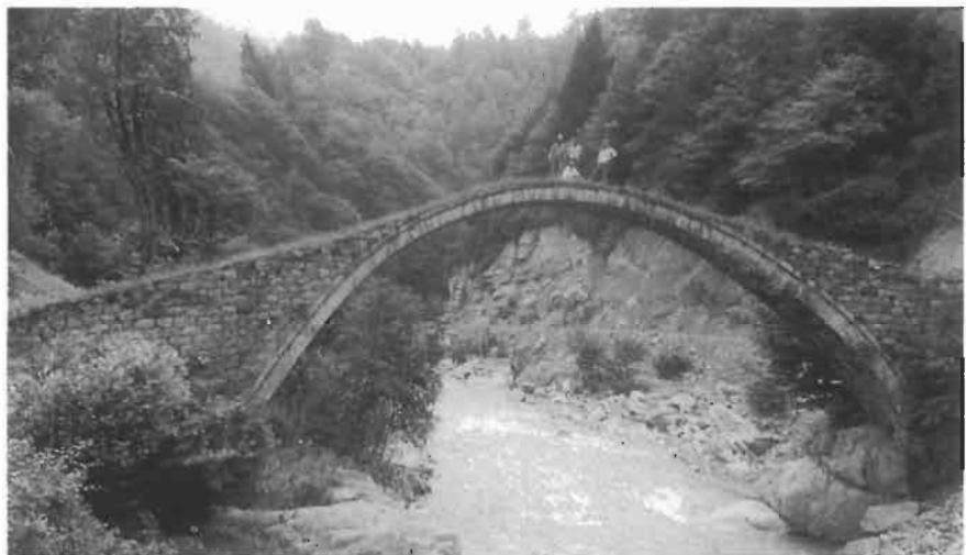
Figure 20.5 Masonry bridge demonstrating a voussoir arch comprised of a single set of rock blocks (northern Turkey).
