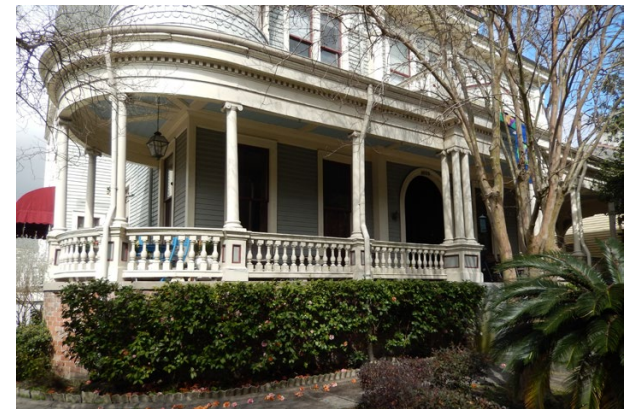
Landscape screening can help buffer parts or almost all of exposed foundations, Lower Garden District, New Orleans (2014)
