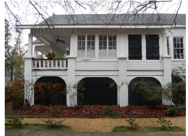
Structural supports take into account the location of prominent features and repeat vertical elements, Covington (2014)
