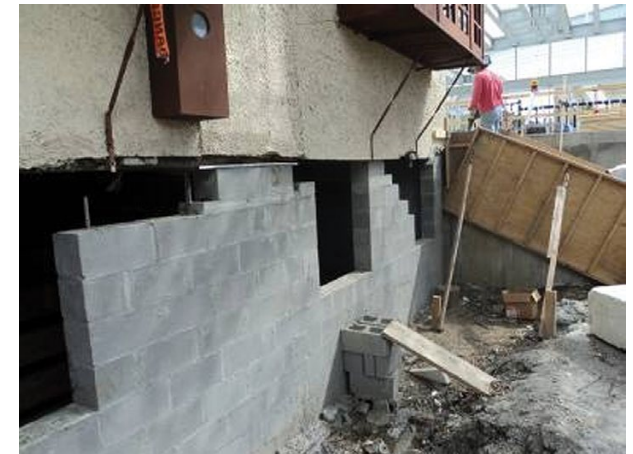
New Foundation at Rosa Keller Public Library, Broadmoor Historic District, New Orleans (2011)
