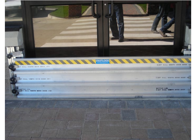
Stackable flood barriers deployed at entrance (2011)
