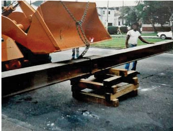
View of steel used to support a house during elevation project on Rampart Street, New Orleans (ca. 1980s)
