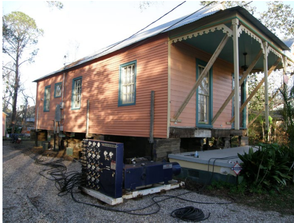
Control panel for unified jacking system, Mar Villa House Guest House, Mandeville (Lynn Mitchell, 2009)
