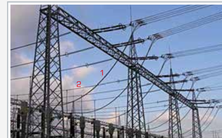
Free-hanging cables in practice (portal): 1 stay cable, 2 power line, similar to overhead line
