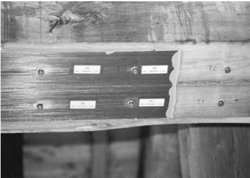
Figure 11.23 The use of bonded gauge studs to monitor long term performance.
