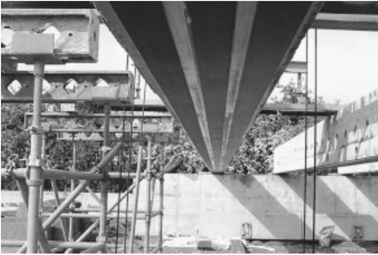
Figure 10.12 Overall view of completed installation of plates to a reinforced concrete bridge beam.
