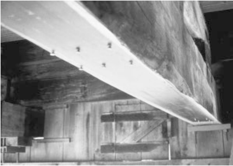
Figure 11.22 A close-up of the bonded plate to the underside of the beam.
