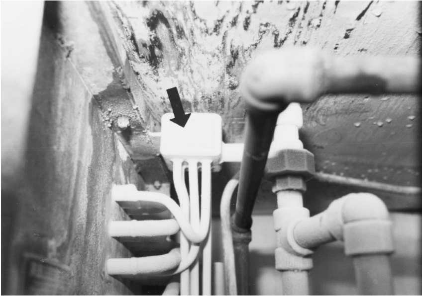
Figure 4.16 The ammonia refrigeration junction, which had been constructed from rectangular tubing, and which failed to stand up to service.
