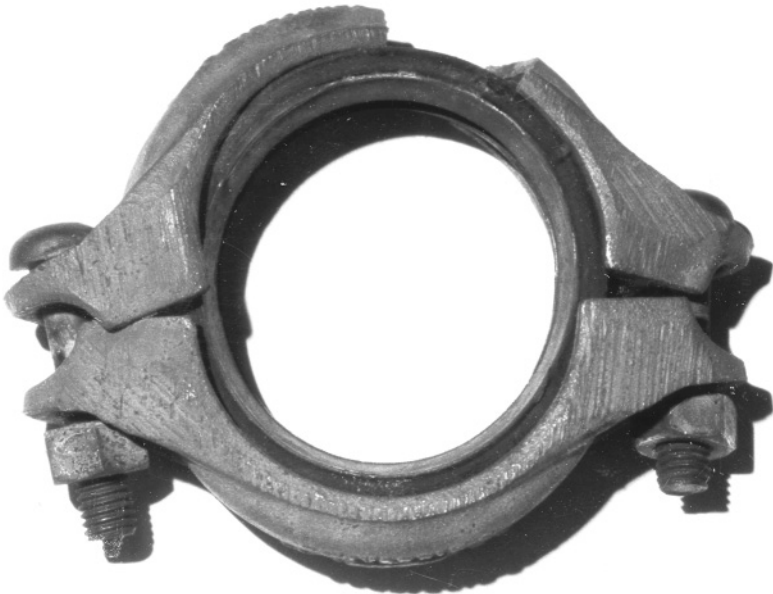
Figure 4.15 The failed coupling that split due to a casting fabrication problem.
