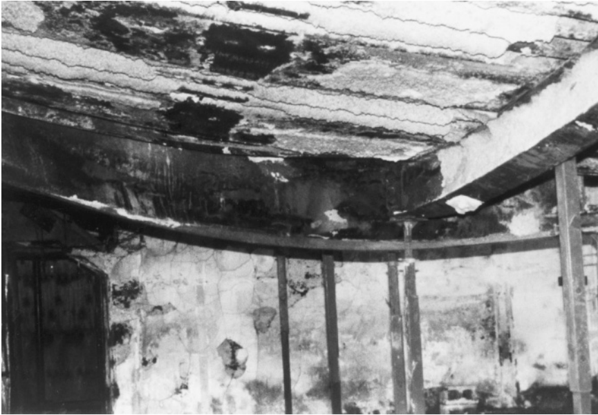
Figure 8.8 Fire damage to steel and concrete floor structure.
