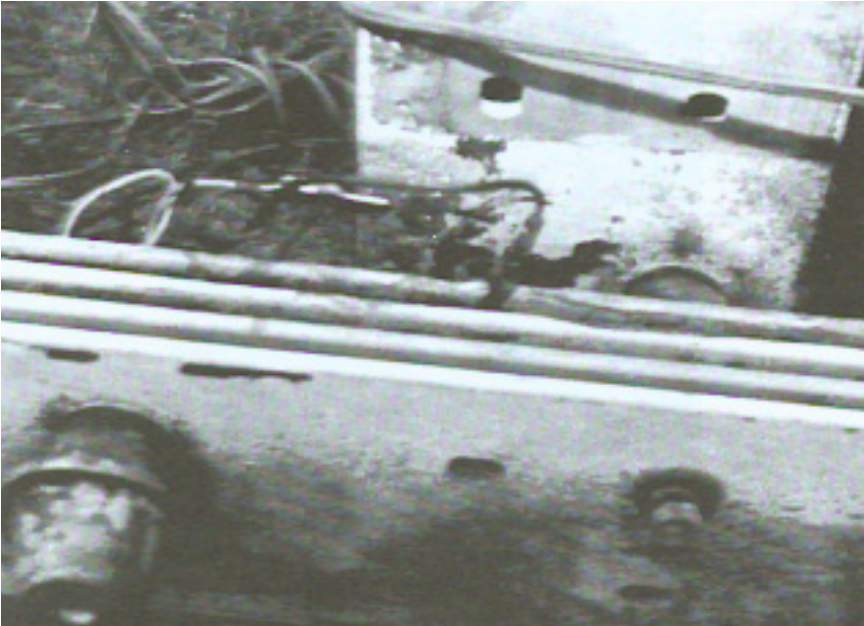
Figure 3.3 Section of switchboard bus grounded by contact with tool.
