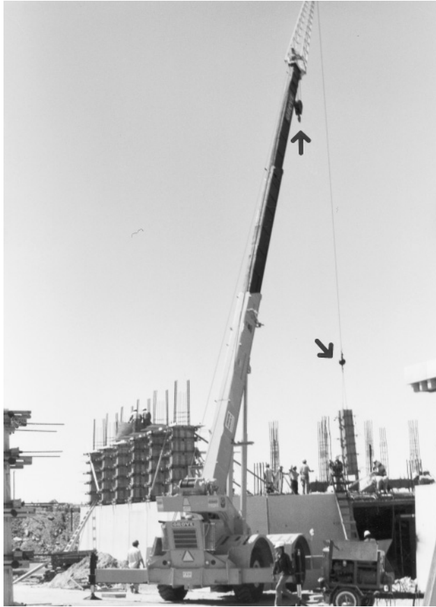
Figure 4.18 The extendible boom crane in use. Note the two cable and block systems, with the outer one being in use at this time.
