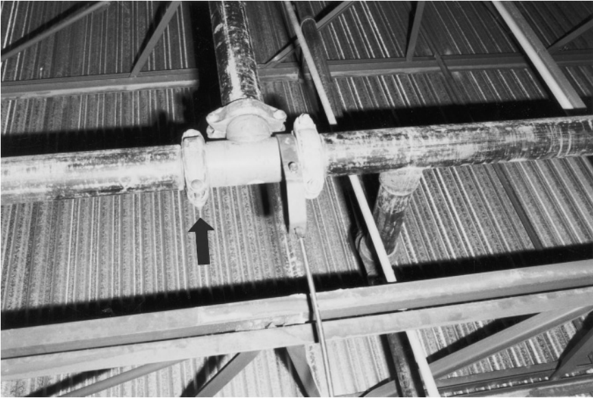
Figure 4.14 Area where a water coupling failed, allowing high pressure water to damage a building containing paper products. The arrow indicates the replacement coupling.
