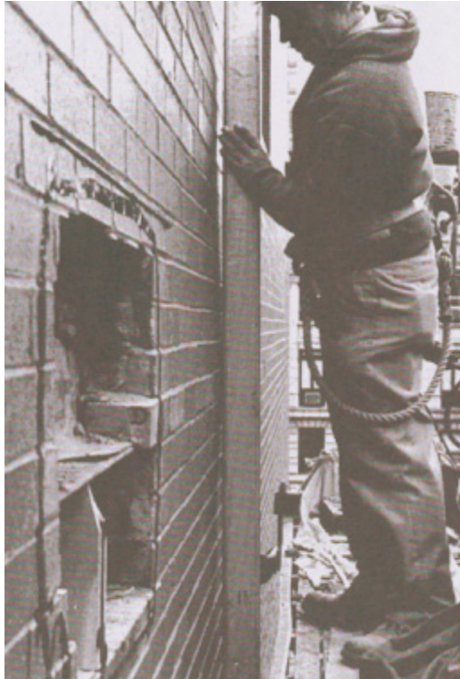
Figure 8.6 Investigation of brick veneer wall bulging at shelf angles.
