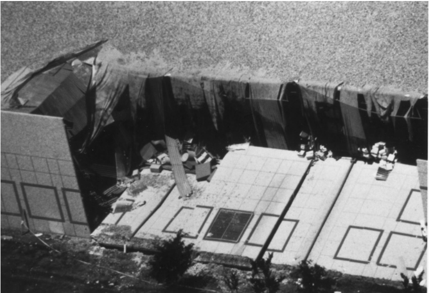
Figure 8.3 Roof and wall collapse from rain-water ponding.
