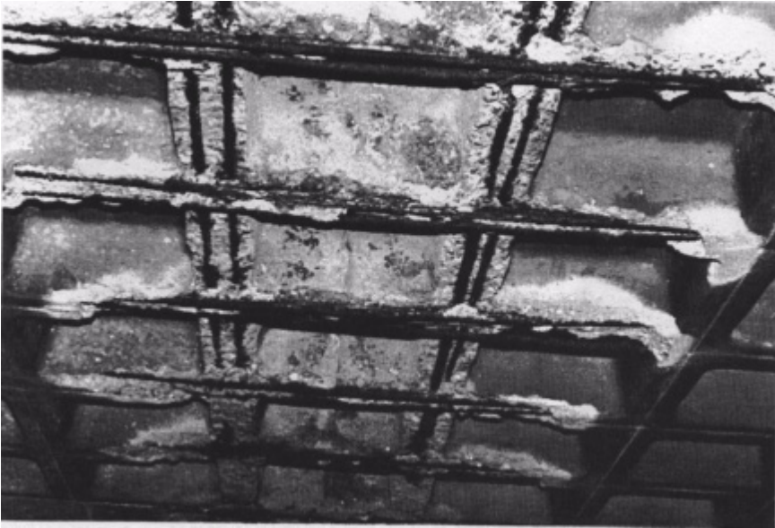
Figure 8.4 Severe deterioration at underside of parking garage slab.
