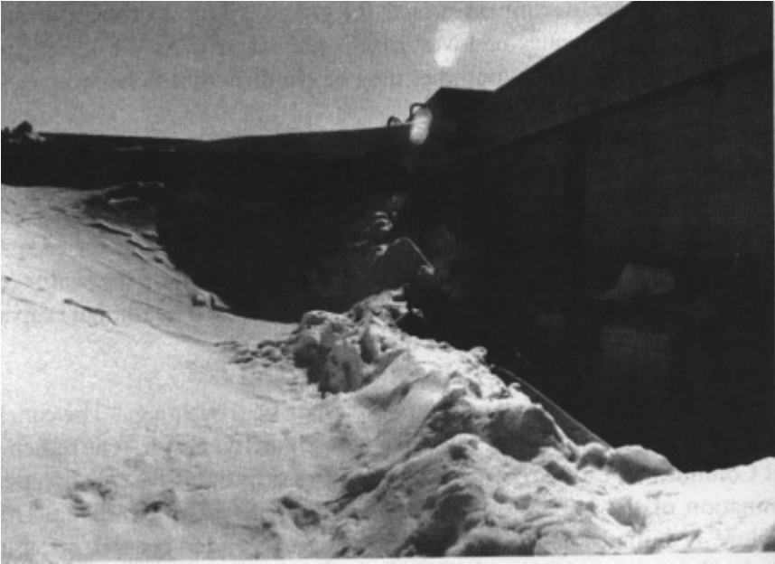
Figure 8.22 Roof collapse under drifting snow, shopping mall, Ohio.
