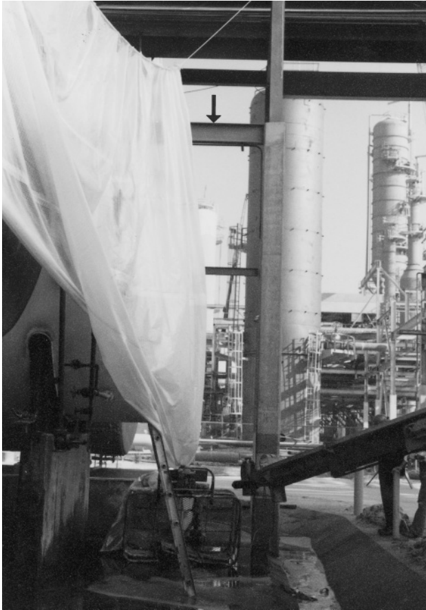
Figure 4.5 Fallen aerial platform basket. The basket separated from its boom connection after coming into contact with the cross beam at the arrow.
