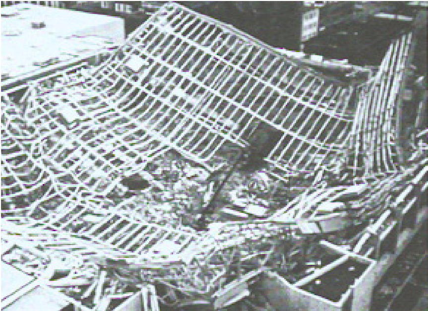
Figure 2.3 Civic Center Coliseum failure, Hartford, Connecticut, 1978. Failure occurred five years after completion. (Courtesy W. Turek.)
