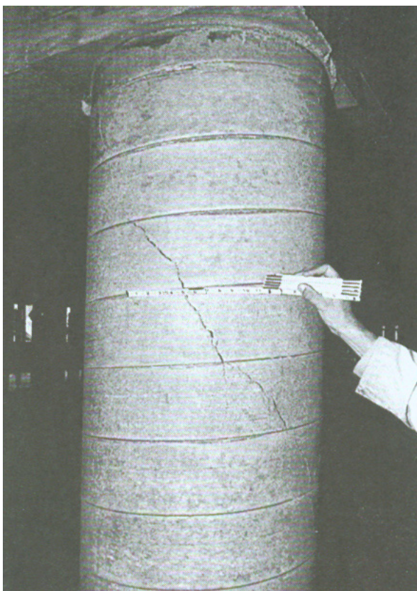
Figure 8.7 Cracking of columns in prestressed concrete garage, Lowell, Massachusetts.
