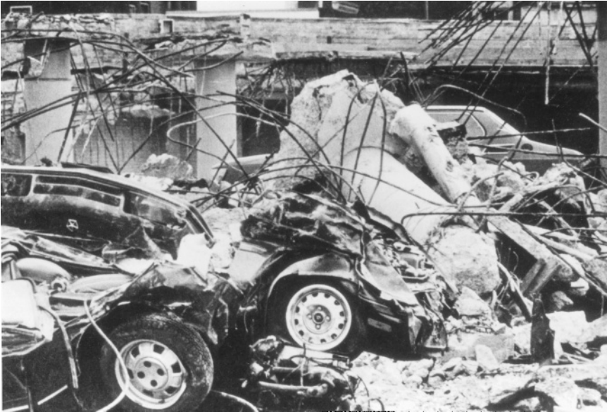
Figure 2.7 Collapse of a parking structure caused by corrosion, concealed beneath a new layer of asphaltic paving. (Courtesy of Rath, Rath & Johnson, Inc.)
