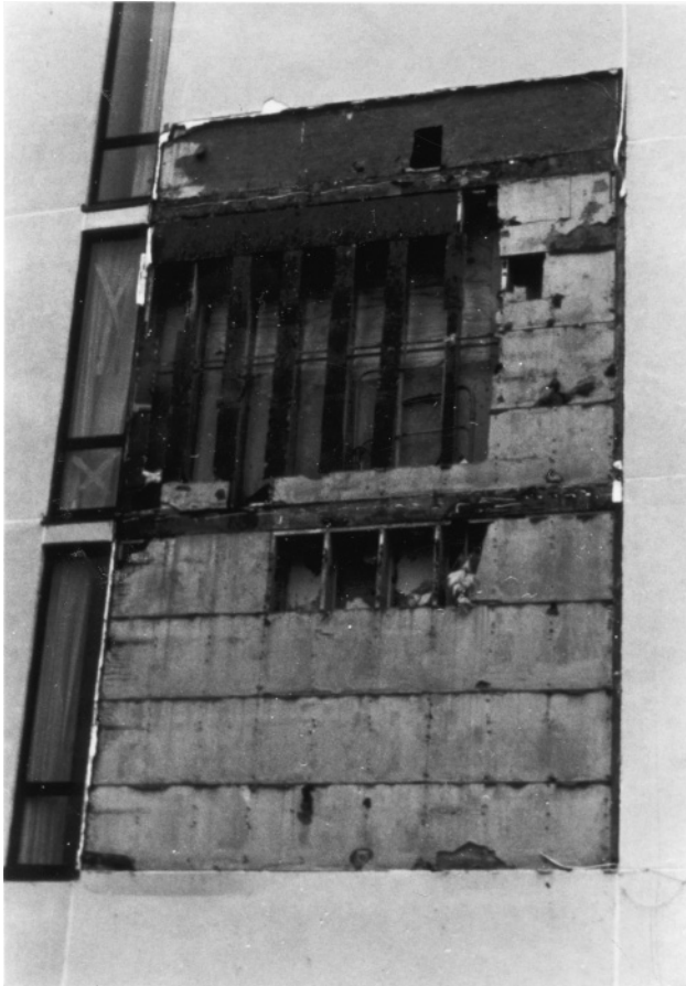
Figure 8.5 Water penetration and long-term deterioration caused loss of wall panels on this building.
