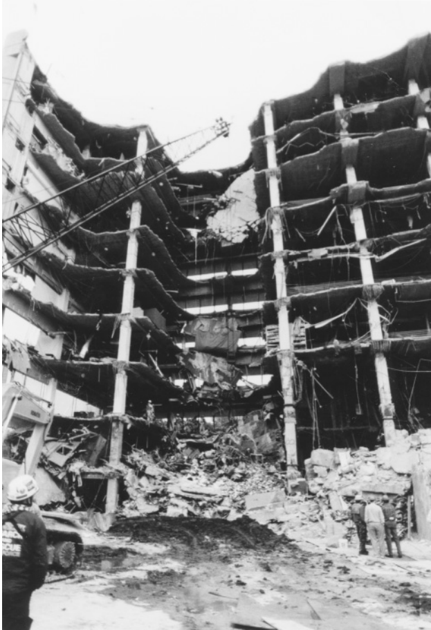
Figure 2.9 Alfred P. Murrah Federal Building, Oklahoma City, Oklahoma, 1995. An intentional act of domestic terrorism claimed 168 lives. (Courtesy of W. Gene Corley and the Federal Emergency Management Agency.)
