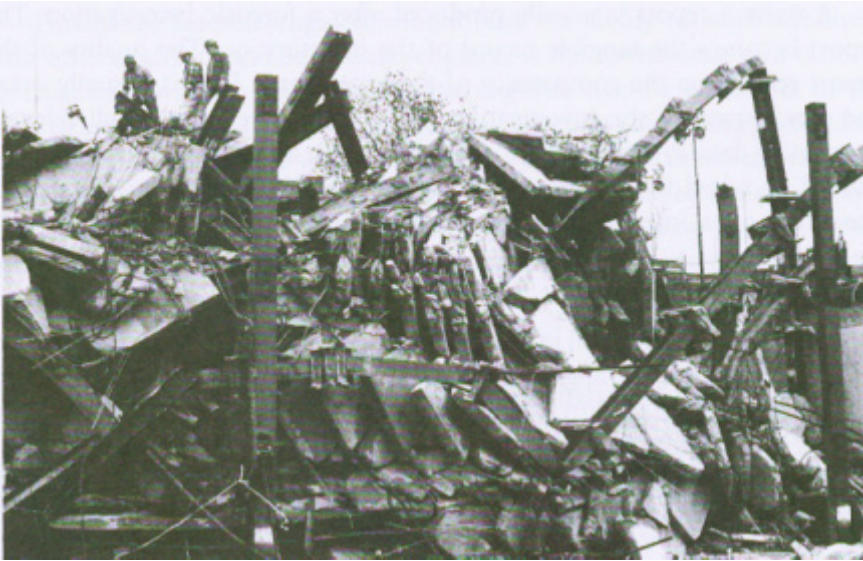
Figure 1.4 L'Ambiance Plaza, Bridgeport, Connecticut. This project collapsed during construction in April 1987, killing 28 construction workers. Useful evidence is often destroyed during the rescue efforts after such an accident [USDC/NBS 1987, Scribner and Culver 1988].
